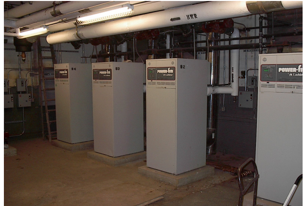
New Modular Boilers
