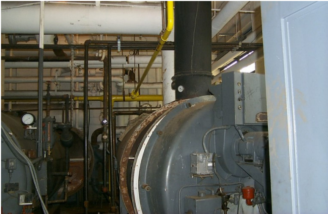
Original Firetube Boilers
